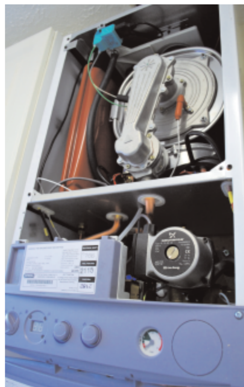
A new Potterton Promax HE Plus 24kw boiler was fitted
