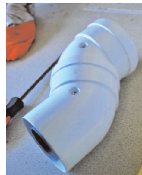
A flue extension was fitted because the flue outlet was in a different place on the new boiler
