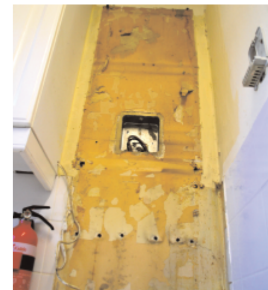
The old boiler and fridge was removed to gain access to the copper pipework
